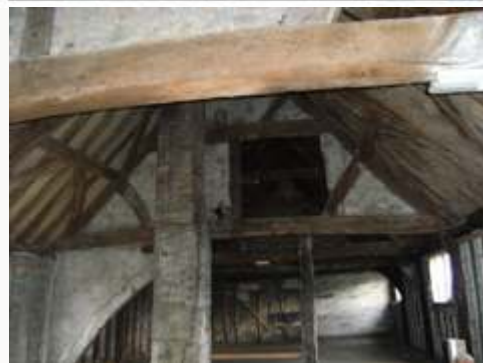
The upper storey of the late-medieval range highlighting the impressive 'cut' roof structure
