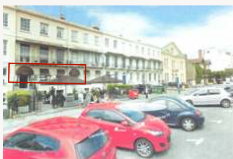
Nos. 9-10 Cambray Place with the two canopies prominent above the entrance doors; note the cluttered and disjointed appearance which is in marked contrast to the clean classical lines of the adjacent period buildings in the terrace
