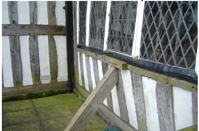
Mere Hall. What happens when you chop an early C19 hole into a C17 timber frame
